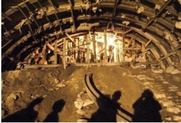
Photograph 1 Treatment of gougy shear zone and 10m high cavity by channel fore-poles
