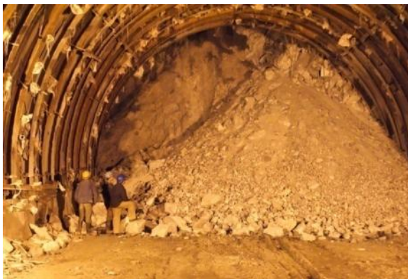
Photograph 2 Shear zone gushing down crushed material and created about 8m deep cavity at crown.
